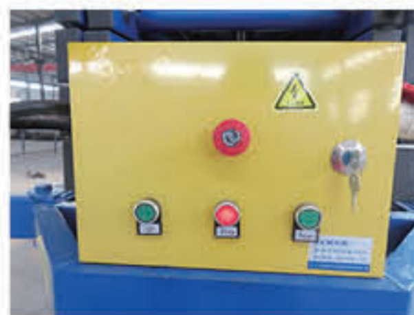
Controller on ground
